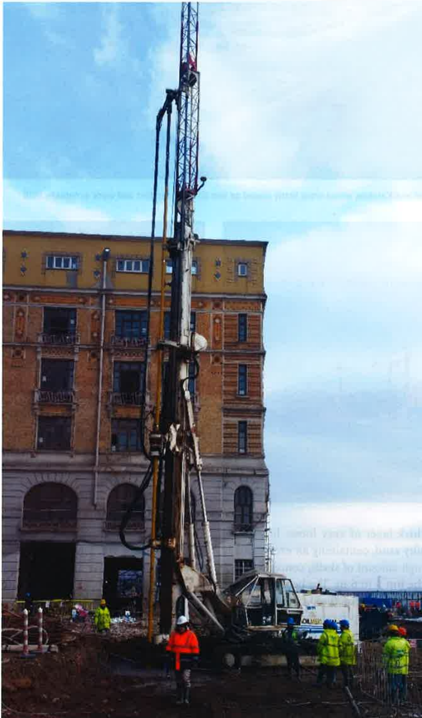
▶ The difficult hydraulic and geotechnical condition required the employment of cutting-edge technologies within the foundation engineering field
